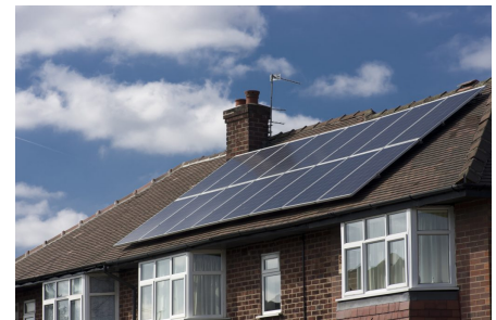
Figure 3: Solar panels can now be seen on rooftops.[22]
